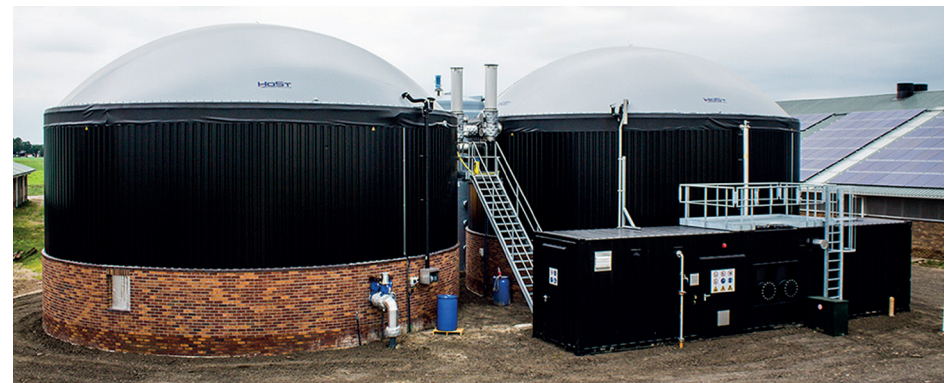
Figure 6 – Anaerobic digester set up in Vrizenen, Netherlands (Source: Host Bioenergy Installations)
