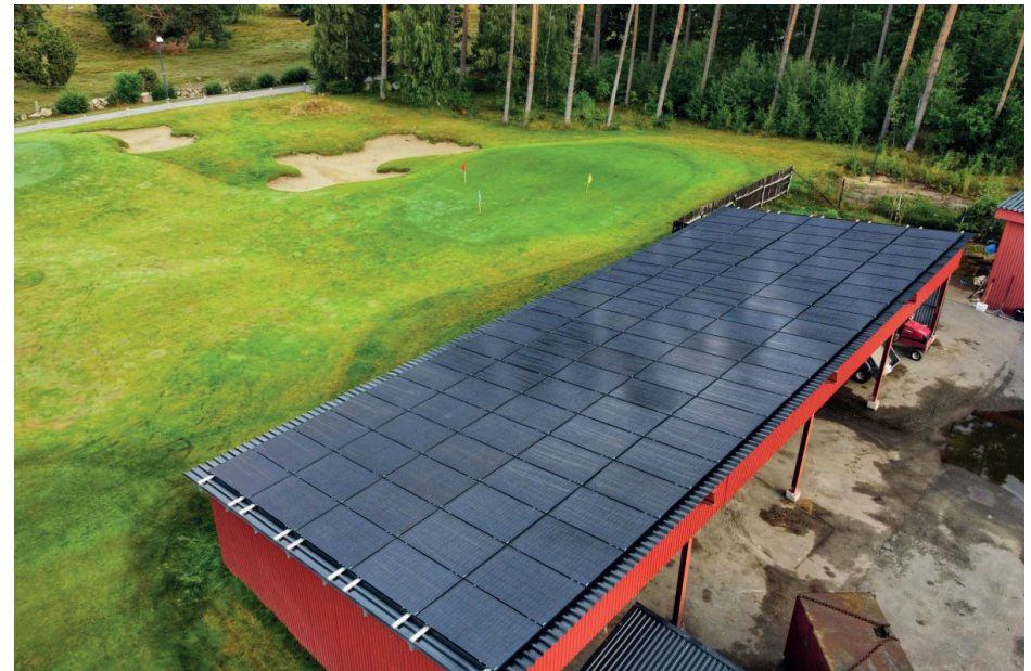
Figure 9. Sölvesborgs Golfklubb, Sweden - ~100kW Solar installation on GMF roof (Source: On-Course® - Highlights)
